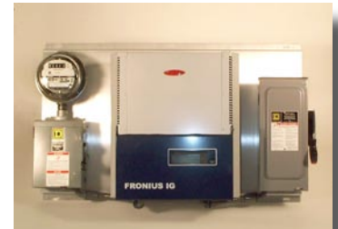
Power Center with Fronius Inverter
